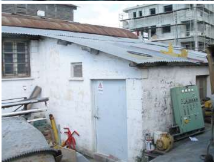
A hazardous chemicals room obviously substandard; allocating "any area" to be a chemical storage room is not a good practice.
