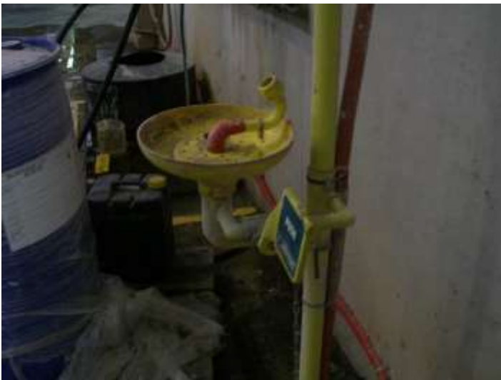
Eye wash station in chemical storage area for one-eyed persons ??? !!!
