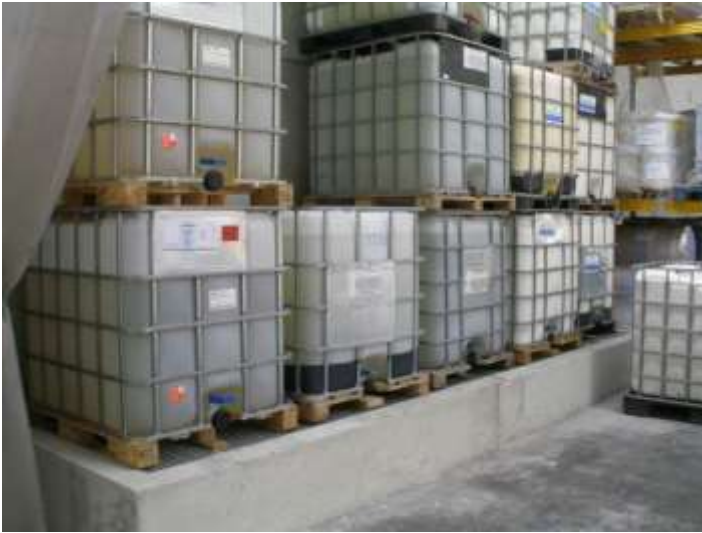
Secondary containment (dike) under IBC's.
