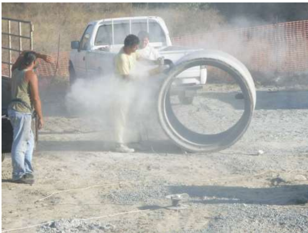
Complete lack of use of PPE during the use of a cement cutter
